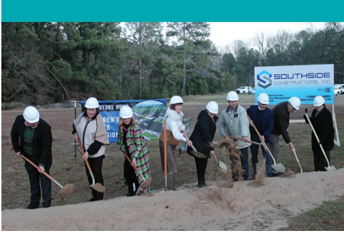
Holy Angels held a groundbreaking ceremony for the Children’s Campus Expansion Project on December 20.
